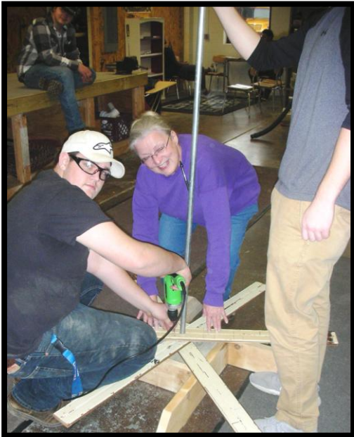
Ryan Watson and Mrs. Biernat are pictured at left constructing a Christmas tree out of salvaged bead board siding.
